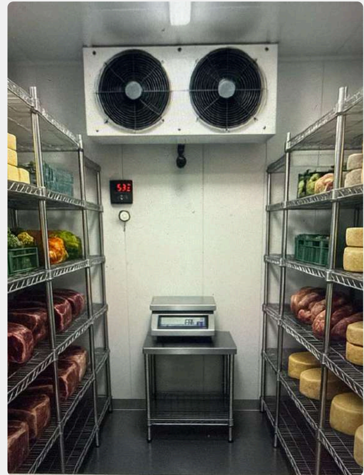
Cuisine stockage walk in fridge kitchen preparation equipment unit n°1 photo de
