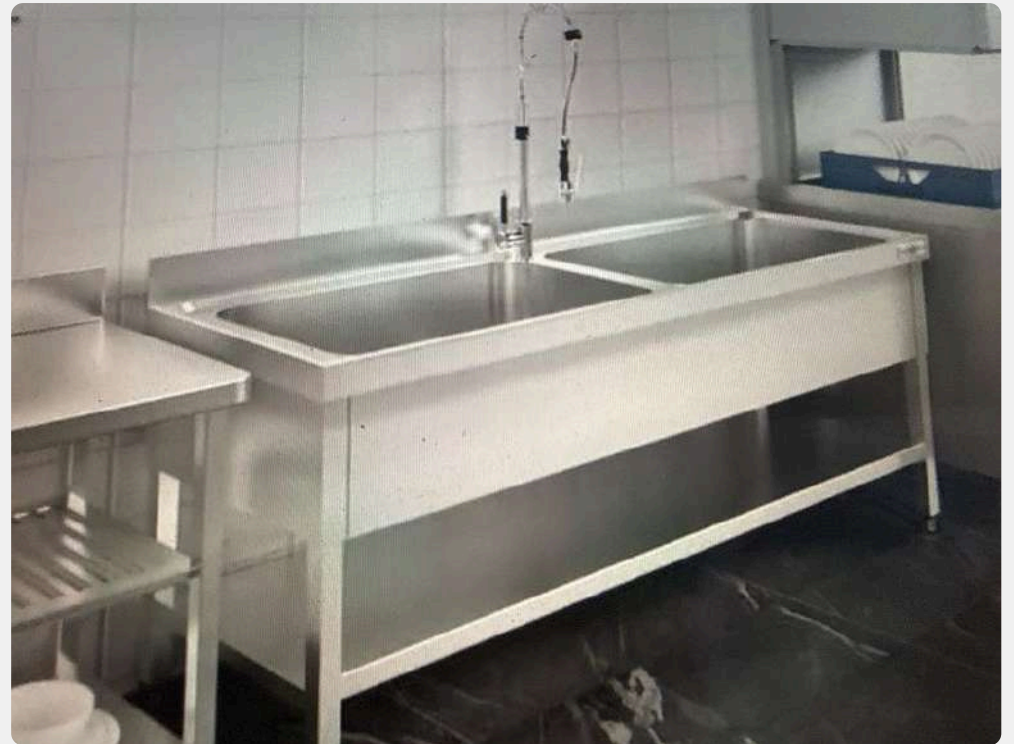
Cuisine entretien pot sink kitchen cleaning and maintenance equipment unit n°1 p
